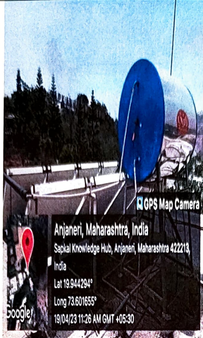
Solar Water Heater
